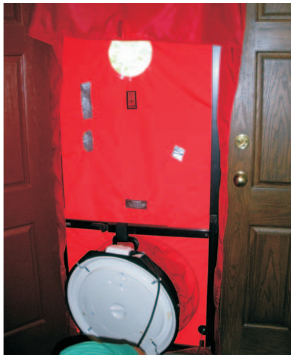
Figure 12: Blower door tests are the most common method to measure air leakage
